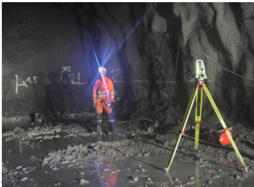
Pic. 5.: Setting out of the theoretical laser for the navigation of the drill rig
